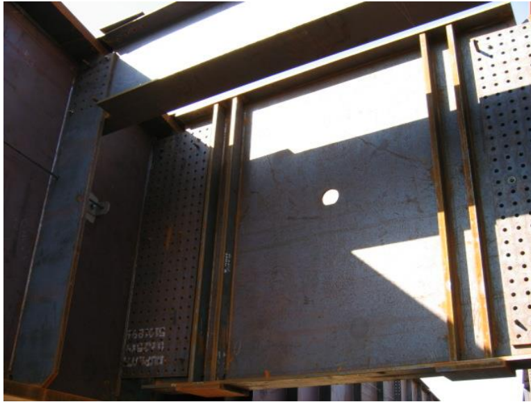
Figure 4 Photograph of a full-depth plate diaphragm at the end of a span
